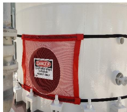
Figure 7 Confined space entry isolation
